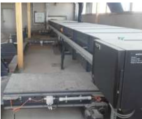
Image 6: The material reaches the storage structure via a chain conveyor.
